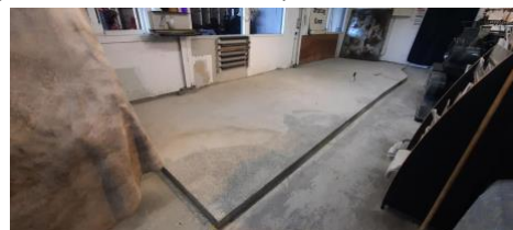
Above: Concrete pad - boxing removed, ready for a clean and a paint
