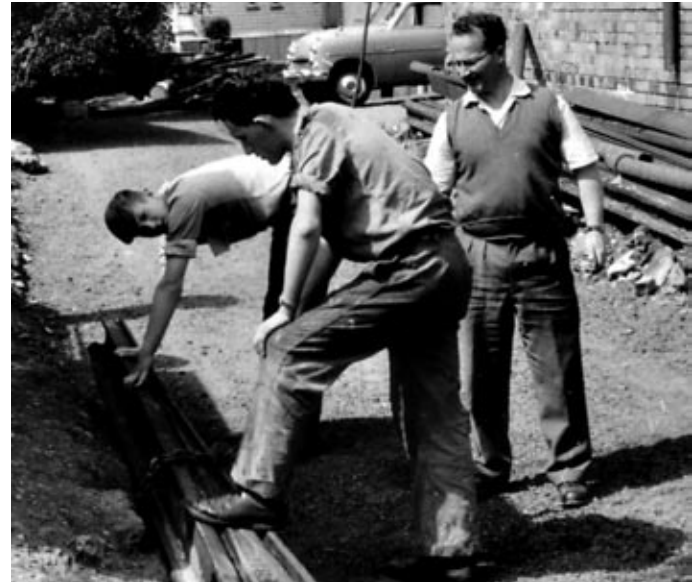
Ian Stewart (right) supervises Ollie Scott (hand on rail) and Ian Jenner, laying a turnout behind the pump house to connect temporary tram storage tracks c.1965.
