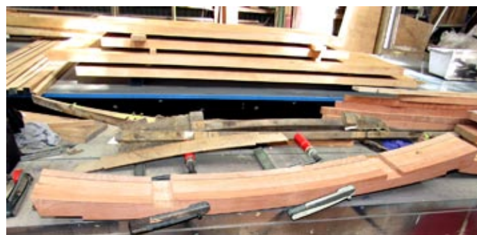
Totara roof bows being worked on in the MOTAT coachwork shop. Behind them are stacks of timber which will form other parts of the body frame.
