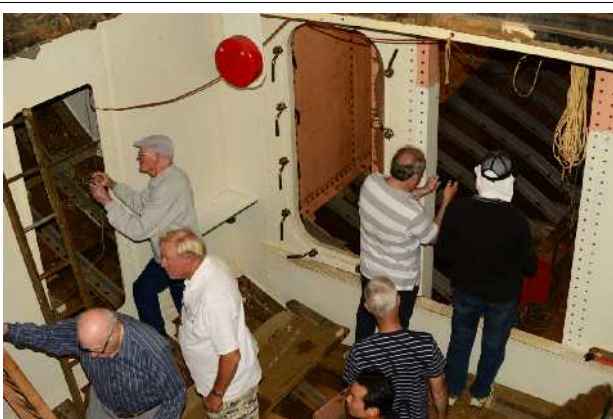
Inside Toroa's engine room - 99% new steel, with bulkheads that will be watertight
