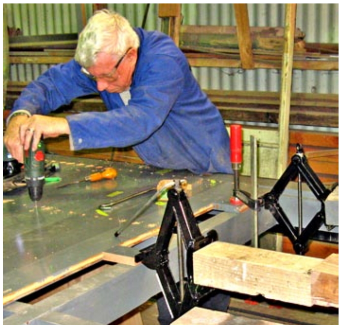
Putting the squeeze on the floor boards of steam tram trailer 21, Paul Warner drills holes through pre-drilled holes in the floor boards to fix them to the underframe. The boards are being squeezed by three car jacks, one at each end and one in the middle, pressing against the end rails of the underframe. Once all the boards are affixed, the holes will be filled with "bog", and the boards will be sanded, sealed and painted.
