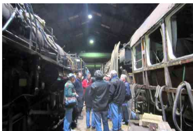
In the top photo, the locomotive to the left is J 1211, undergoing firebox repairs, to the right is a 56ft carriage undergoing restoration,
