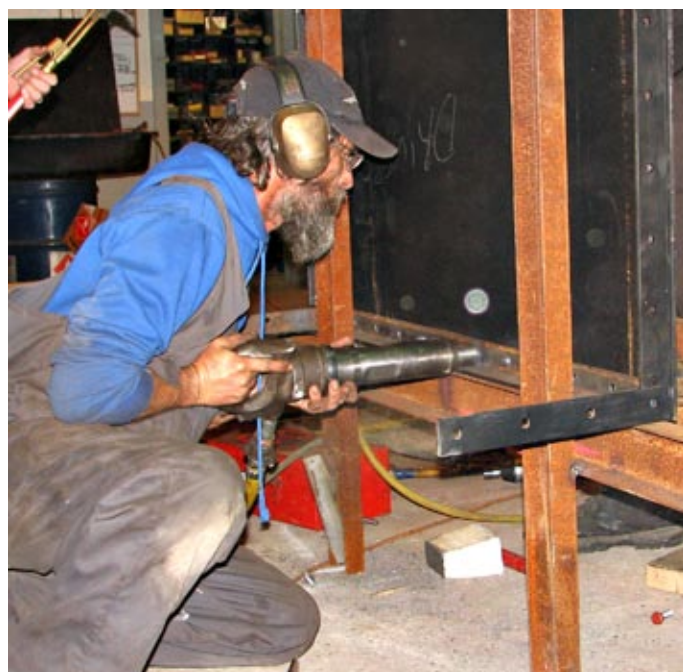
Rail Section's Paul Spearpoint, hot rivetting part of F.180 (Meg Merrilees) cab.
