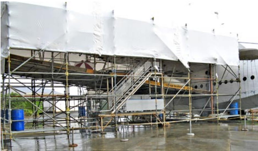
Protection against the weather and safe working conditions are paramount for Aviation Section volunteers working on the Sunderland aircraft.
