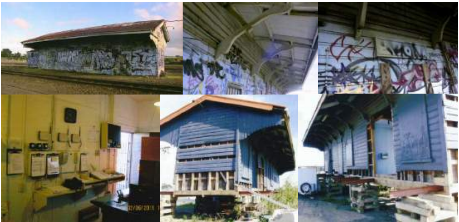
Clockwise from top left: Graffiti Canvas - Wiri Station Building 28 June 2005, Down Main (east) side, looking derelict but housing essential signalling equipment. Closed as a passenger stop, track raised above platform level; Interesting Verandah supports; Wiri Station Name board (Photos: RBC 28/6/2005); Floor joist replacement completed by Papatoetoe Railway Station Trust; Work at a standstill. December 2014 (Photos: Bruce Wild); Wiri building prior to shutting down of signal panel and relocation from between the two Main Lines (Photographer unknown).
